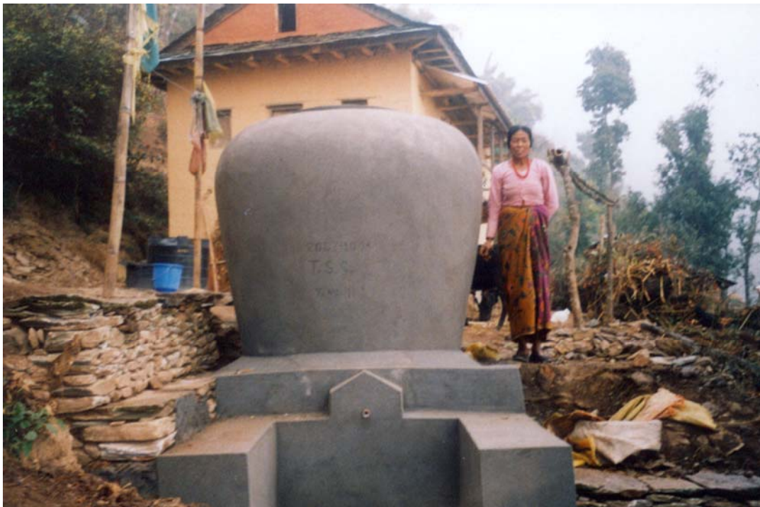
COMPLETED RAINWATER HARVESTING STORAGE TANK
